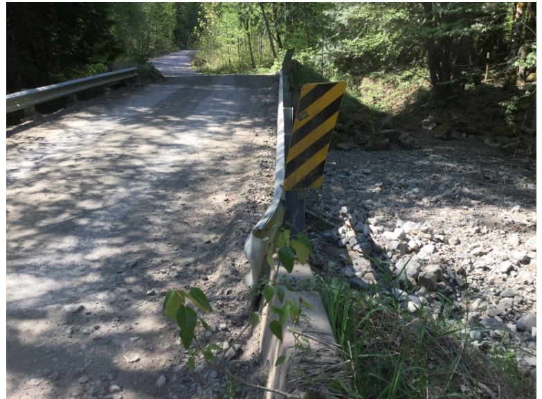
Upstream left approach guardrail condition
