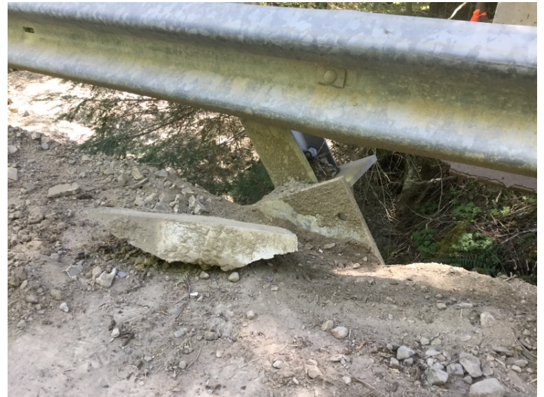
Downstream right approach damage to deck at steel riser location
