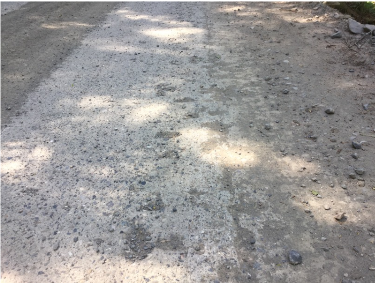
Wear noted on wheel path
